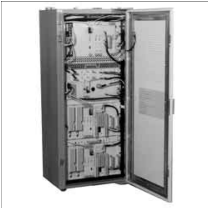
Base station of cellular network
