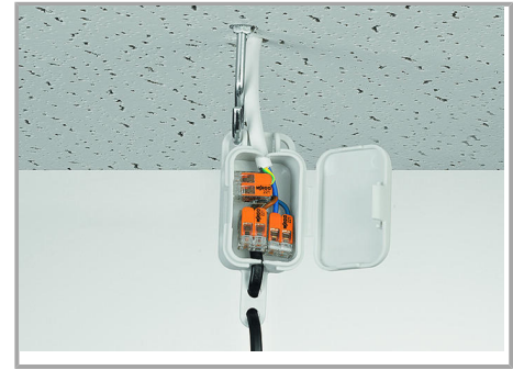
Pendant light connection in suspended ceilings
