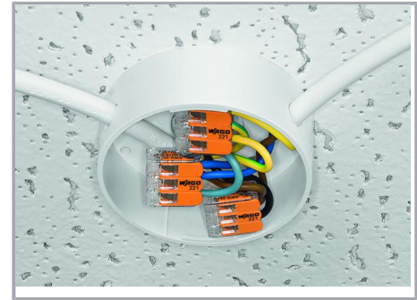
Lighting distribution in a ceiling canopy
