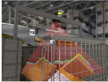
Figure 2. ZMX Sensor and Tower Light At the Bottom of a Chute
