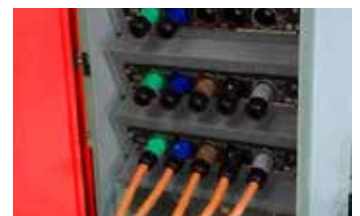
Emergency power systems
