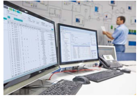
Remote control: secure and continuous transmission of process data to the control center
