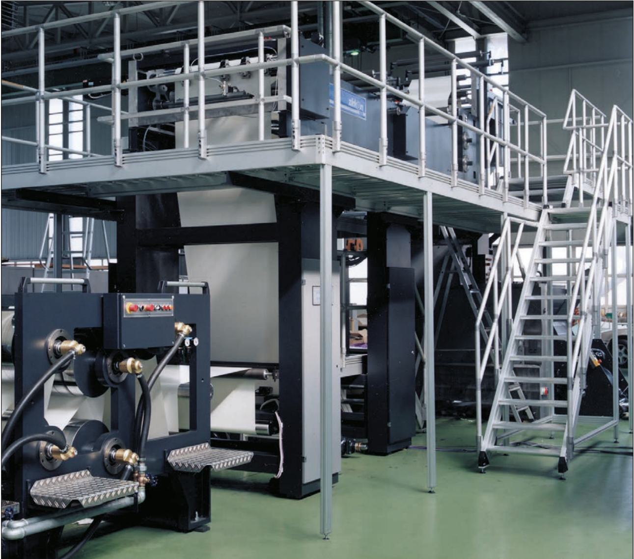
Platform with staircase on a web offset machine.
