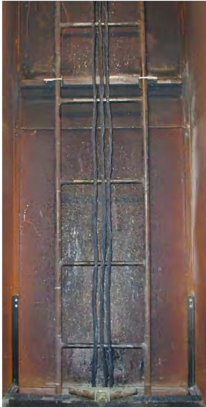
Photo 1: Cables before test
