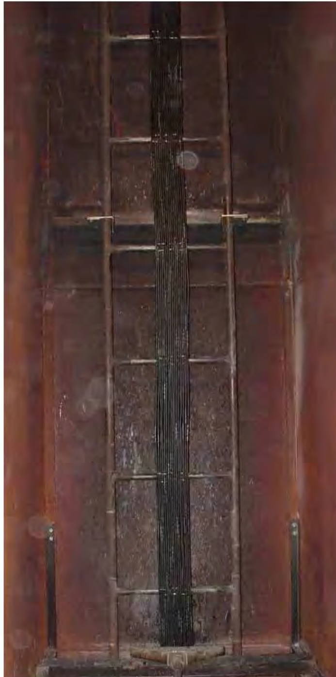
Photo 1: Cables before test
