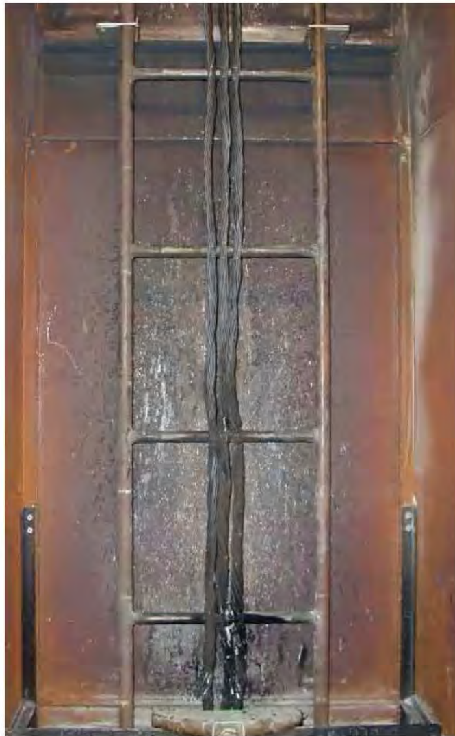
Photo 2: Cables after test.
