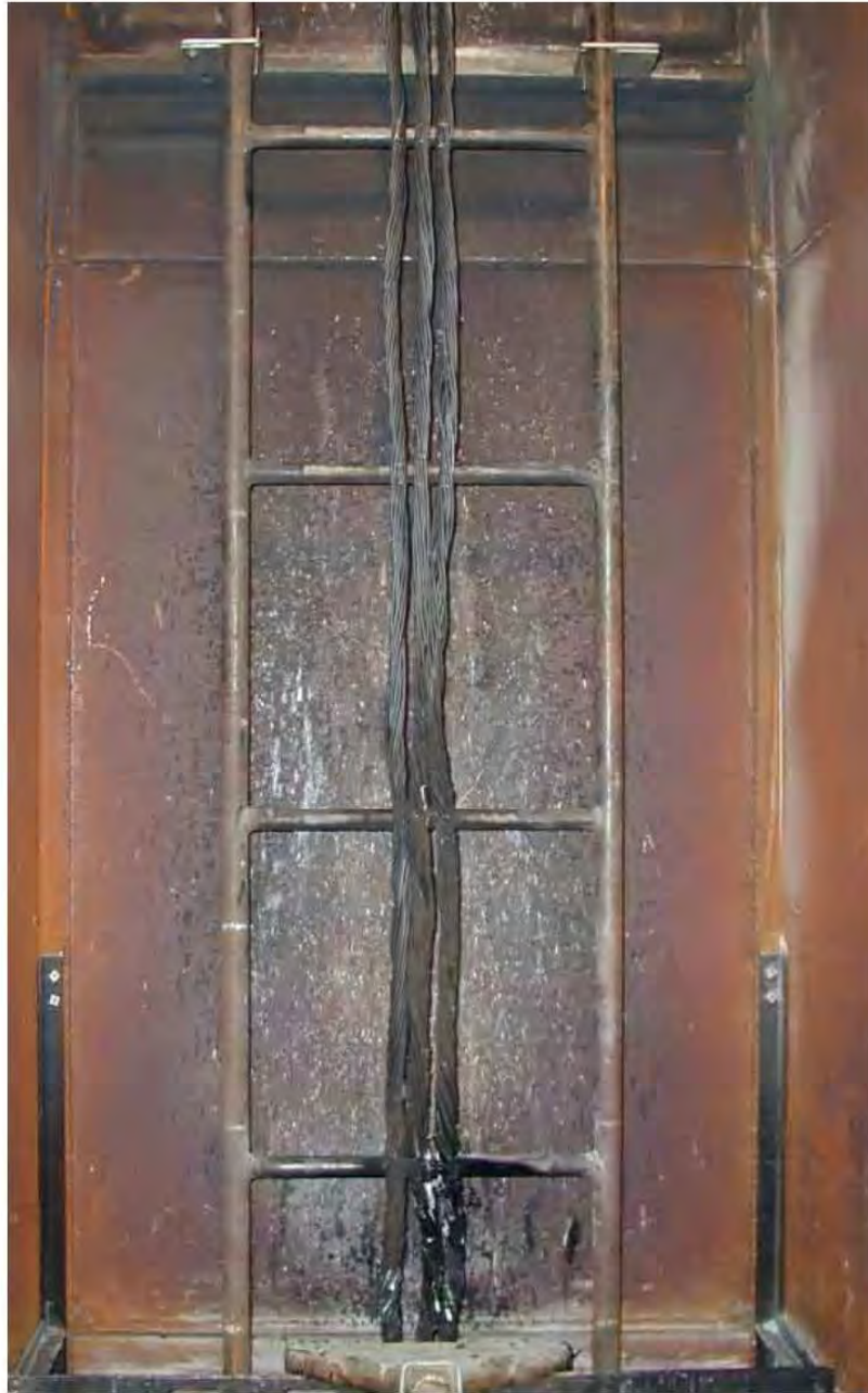
Photo 2: Cables after test.
