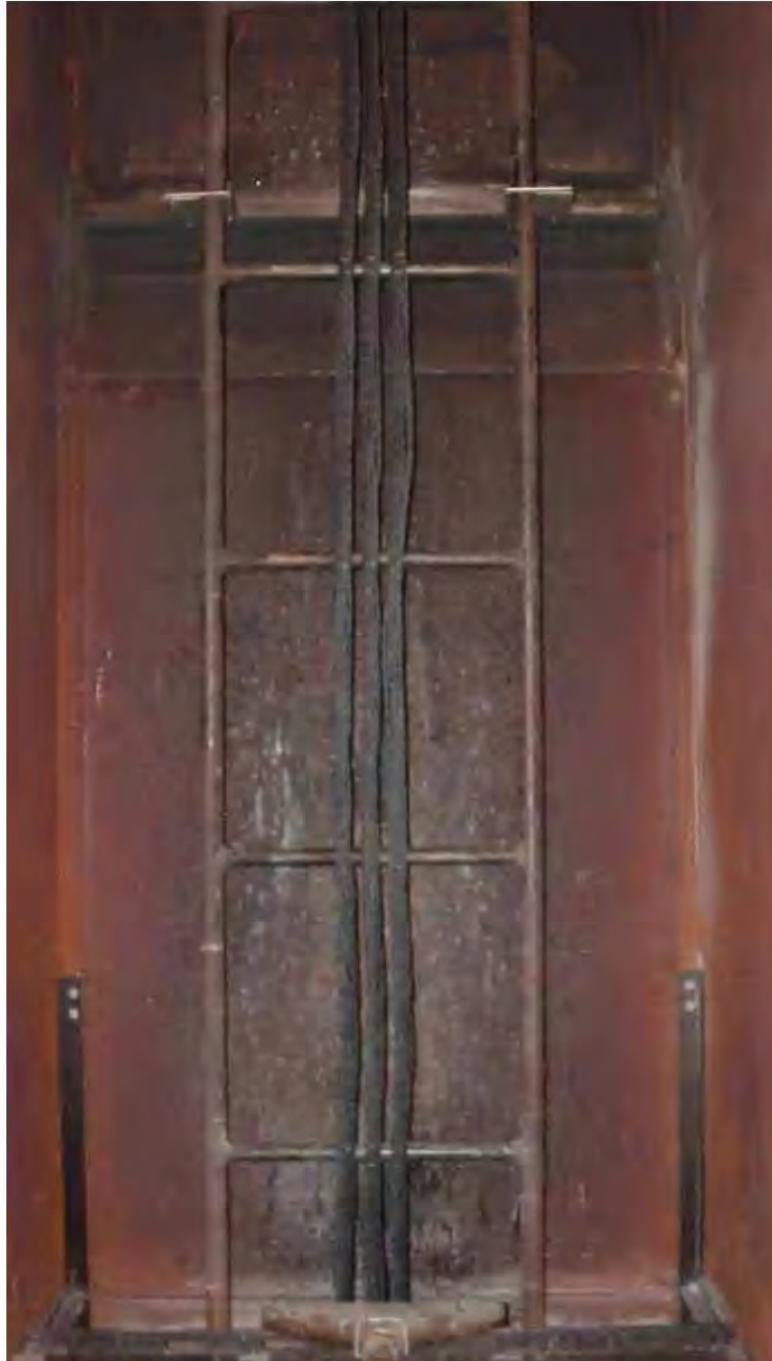
Photo 1: Cables before test
