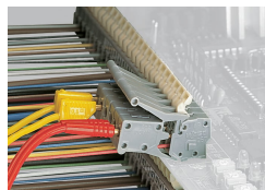
Testing with test plug modules.
