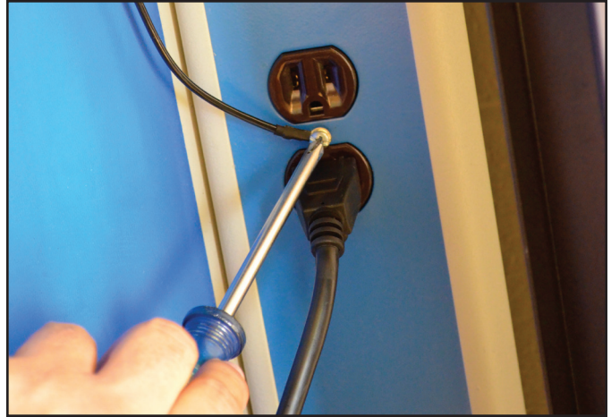
Figure 8B. Grounding the SCS 724 Workstation Monitor
