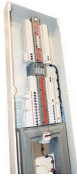
Vertical split-load board
