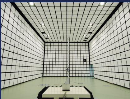
RF anechoic chamber
