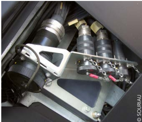
Closed electrical areas
