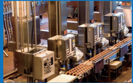
Distributed Monitoring and Control Systems
